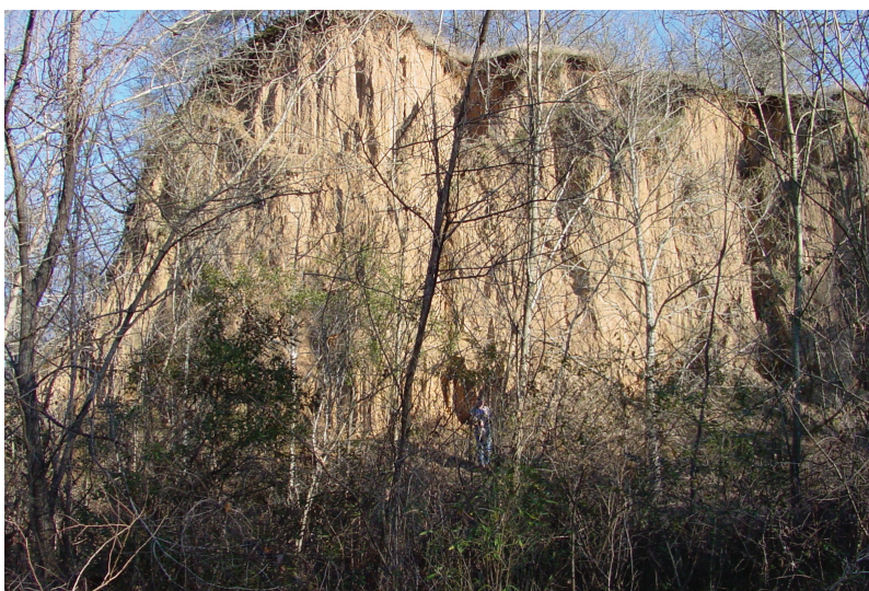
Figure 4. Loess cliff on edge of former gravel pit, Sicily Island Hills, Catahoula Parish, Louisiana. Estimated height of cliff is approximately 45 feet high. (Photograph courtesy of Mr. Richard P. McCulloh)
